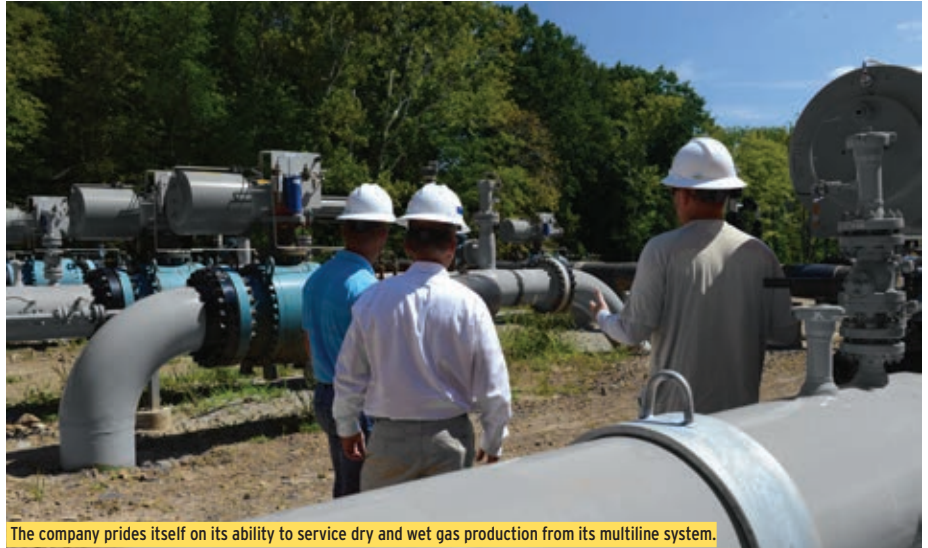
The company prides itself on its ability to service dry and wet gas production from its multiline system.
